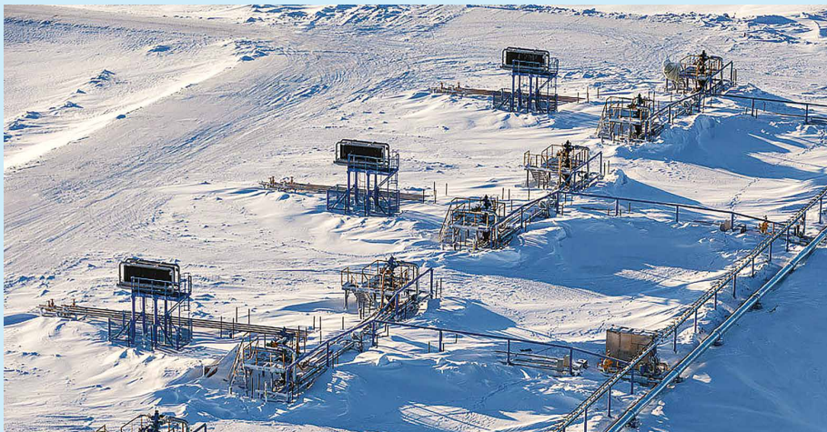
The VET soil temperature stabilization systems at the base of gas well clusters of the Bovanenkovskoye field.
